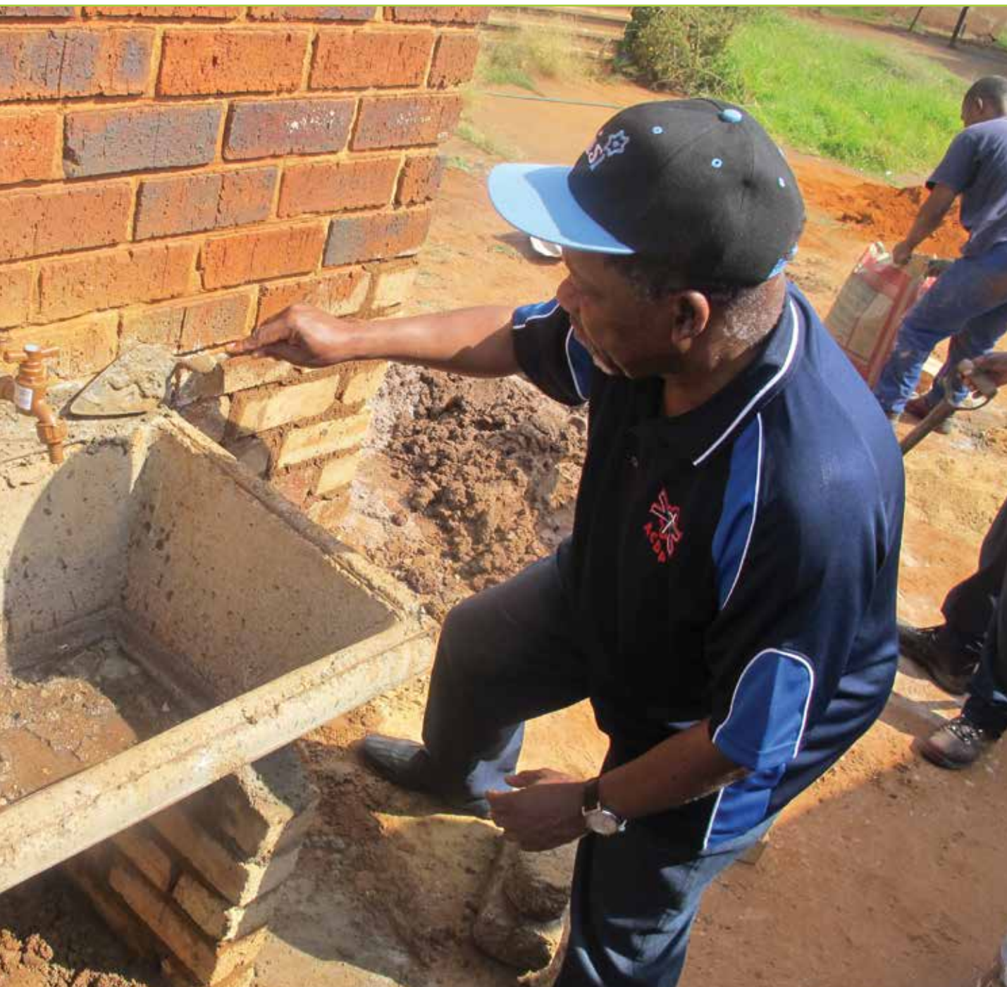
HELPING HAND: Rev Kenneth Meshoe helps to install a communal washbasin in Katlehong in Gauteng.
