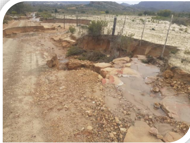
Road damages, W Coast
