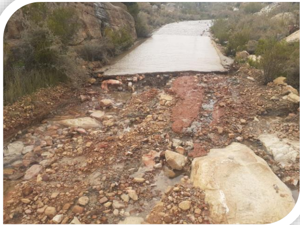
Road damages, W Coast
