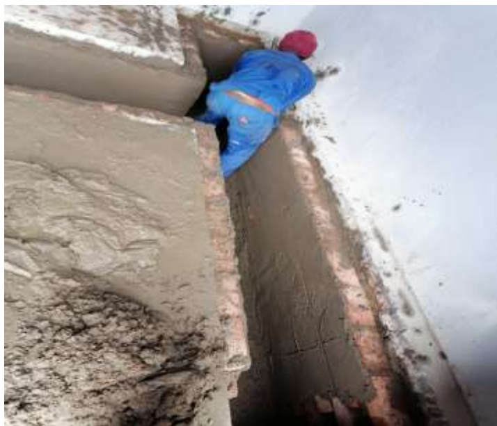
MCC electrical cable trench.
