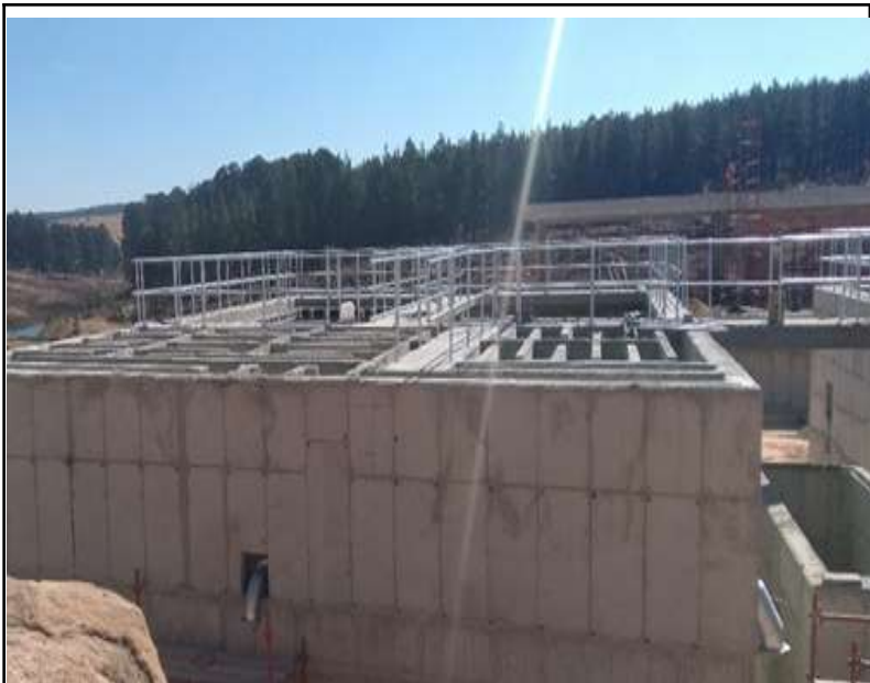
sedimentation and flocculation channel.
