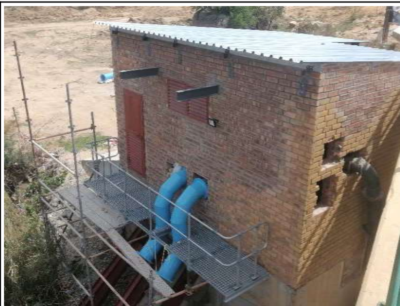
Two suction pipes.
