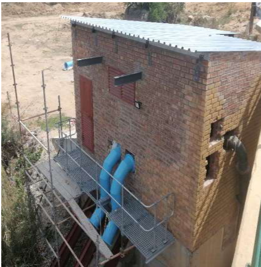
Two suction pipes.
