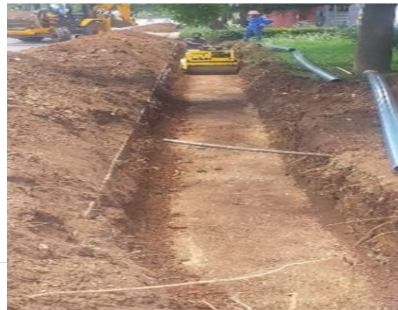
THWS: Ekgangala sewer
