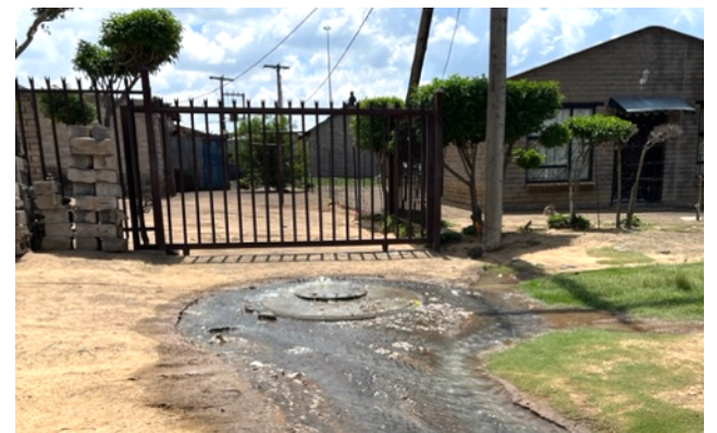
Poor maintenance. and broken infrastructure are frequent and great concern to many communities
