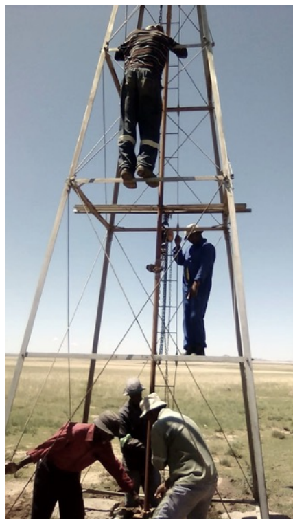
Some of the farmers fixing a windmill for water supply to both livestock and crops in Gladstone.
