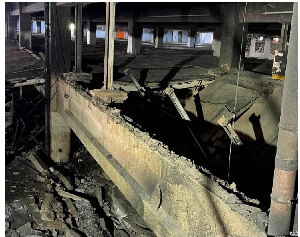
Figure 10: Collapsed 3 rd floor slab area
