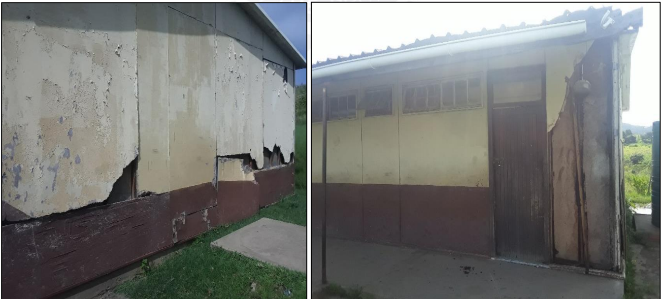
Figure 1: Tekwini JSS state of the buildings
