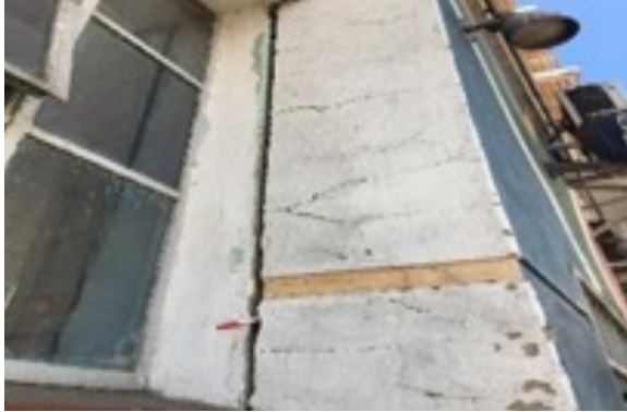
Police station – cracked column
