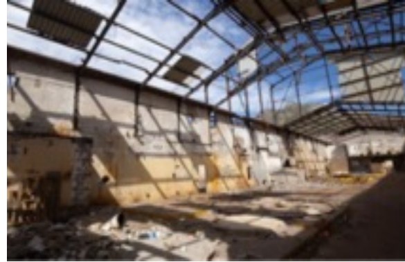
Fishmeal factory – abandoned and stripped by looters
