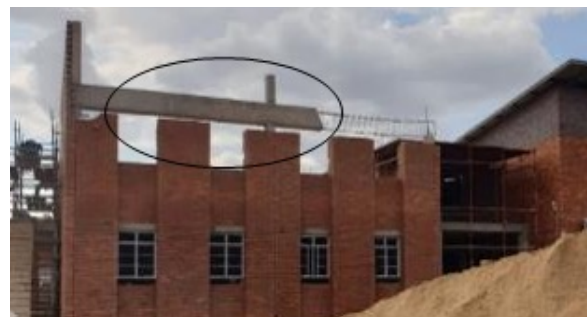
Inadequate load-bearing columns for span of concrete floor slab above
